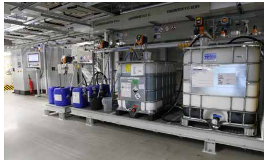
Automatic dosing unit
