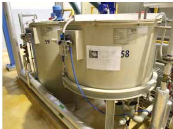
Chemical preparation unit
