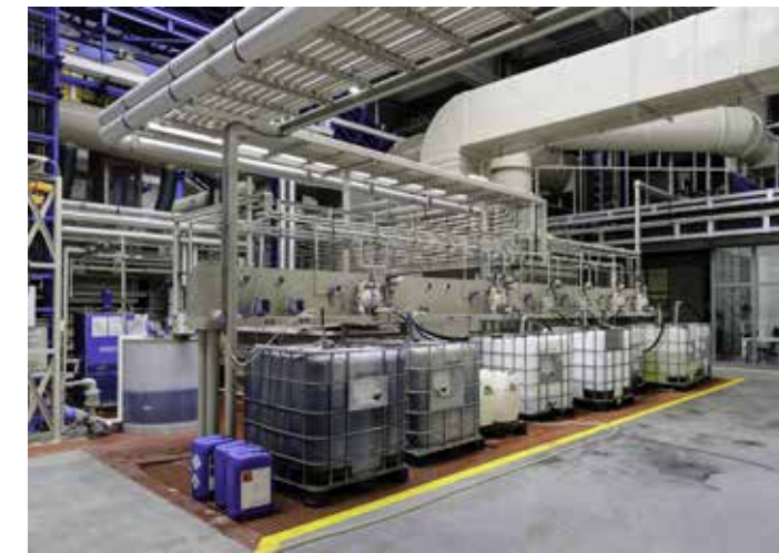
Automatic additive dosing unit
