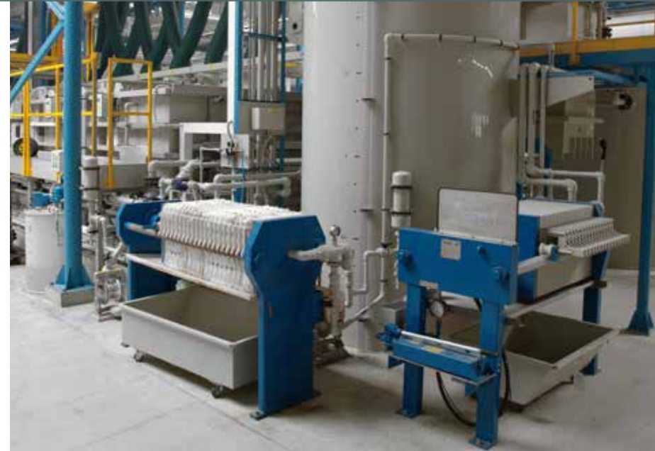
Sludge removal system
