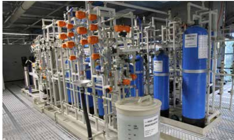
Circulation ion exchanger
